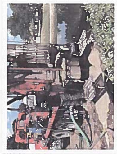
4" Recharge Well - Portsmith & Corinth
