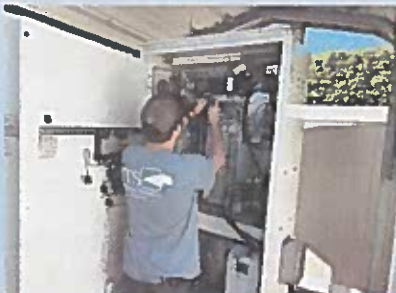
Upper Loop 40Hp Pump Station Retrofit
