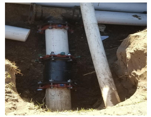
6" mainline break at Hassel Park
